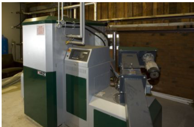
National Forest Youth Hostel 95kW boiler
